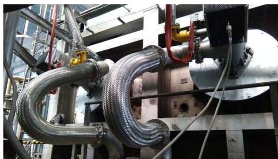
Obr.5: Nový stav anódovej pece, po horákov Oxipyr®-Air New state of anode furnace, after installation of two Oxipyr®-Air burners
